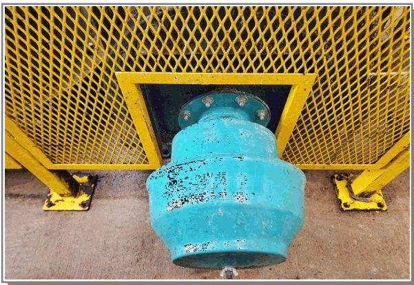
Combustion Blower Air Inlet
