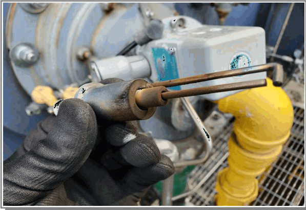
Spark Igniter (Dirty)
