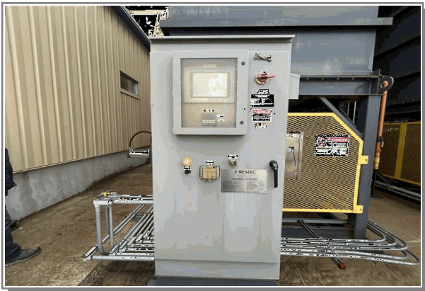
Main Control Panel
