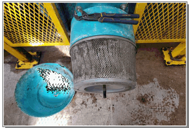
Combustion Blower Air Inlet
