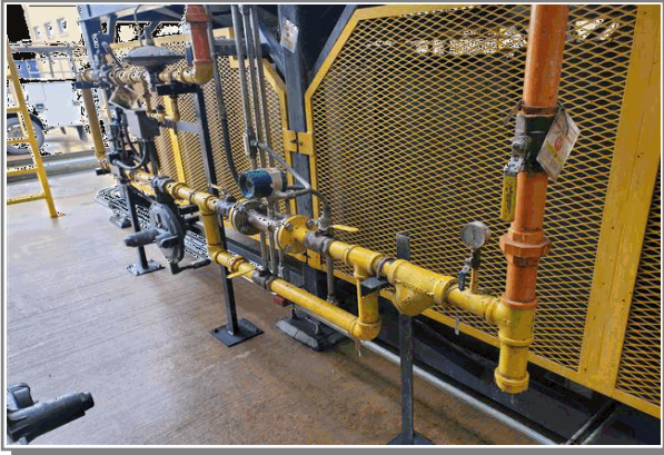
Main Valve Train
