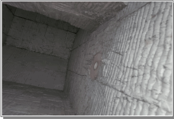
Internal Combustion Chamber & Burner Cone
